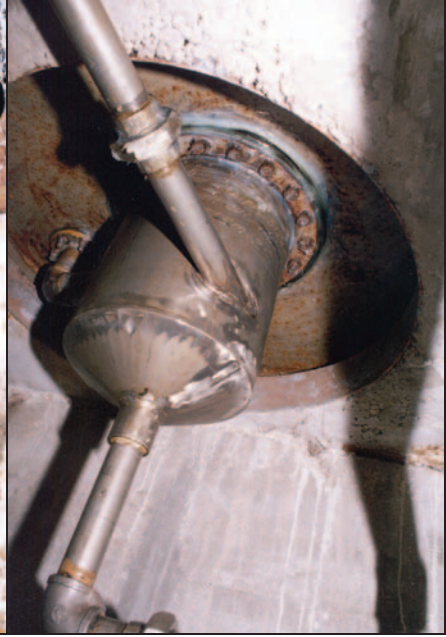
Fig. 104: View of stainless-steel plumbing and chemical container directly under seat in gas chamber.
