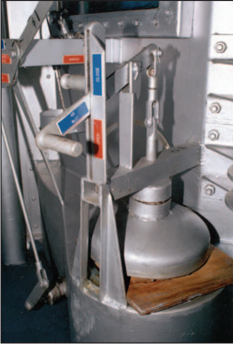
Fig. 95: Closeup of fresh-air intake of gas chamber.
