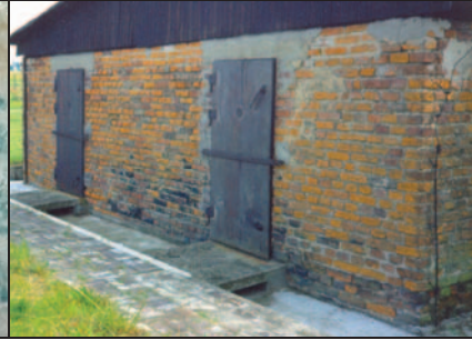
Fig. 42: Blue staining of the Zyklon B disinfestation installation, Chambers II and III (exterior wall), of Barrack 41 in Majdanek Camp. (© Carlo Mattogno 227 )
