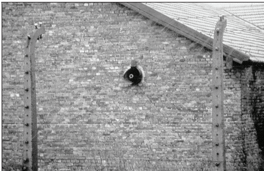
Fig. 24: One of the two ventilation outlets from the disinfestation wing of Building BW 5b, without equipment today. The other is located on the same wall slightly to the left. The end of a water pipe installed after the war is protruding out of the hole.
