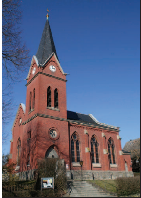
Fig. 35: In August 1976, the Protestant church at D-96484 Meeder-Wiesenfeld was fumigated with Zyklon B. Subsequently, blue-colored stains appeared all over the plaster (see Fig. 36).
