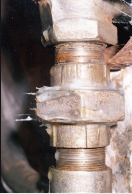
Fig. 103: Closeup of plumbing underneath the gas chamber covered in Vaseline to indicate leaks.
